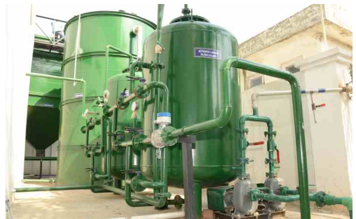
STP at Trikuta Bhawan, Katra.
